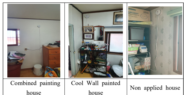
Fig. 7. Combined painting, cool wall painting, non applied house – indoor IoT equipment installation
