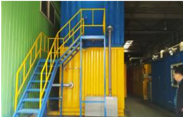
The view of full-scale pilot ( P City facility management corporation )
